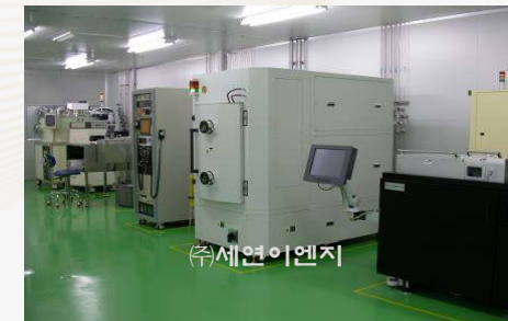
UTILITY HOOK UP
